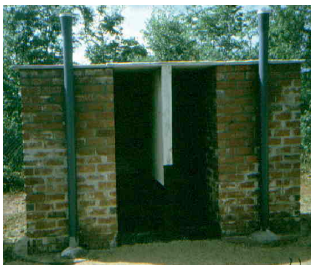
Figure 3.16: Double-compartment VIP latrine at a rural school in Zimbabwe: one side for girls, the other for boys.
