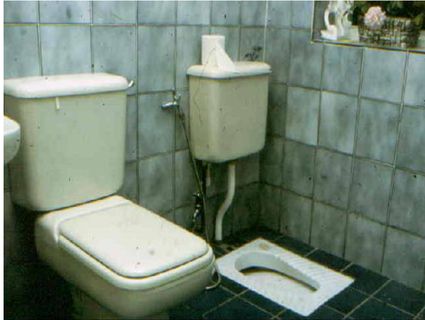
Figure 3.15: The toilet in a house in Bradford, England, belonging to an Asian doctor who has some family members and friends who are sitters and some who are squatters, so he installed both a pedestal-seat unit and a squat-pan unit. Notice the flexible water pipe and tap between the two units and the toilet paper on top of the squat-pan cistern – provision for both washers and wipers.
