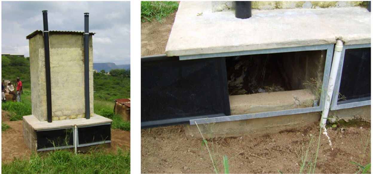
Figure 3.4: An eThekweni latrine – top left: front view showing the urine-diverting pedestal seat unit, urinal, and cover over the entrance to the vault not in use; top right: close-up of the urine-diverting pedestal seat unit; bottom left: rear view showing the two vent pipes (one for each vault) and the small urine pipe (in the centre) which leads to an adjacent soakaway; bottom right: close-up of one of the two vaults with the sliding door open showing the dehydrating vault contents.
