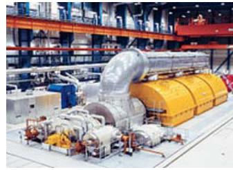
Gas turbine (courtesy of Siemens)
