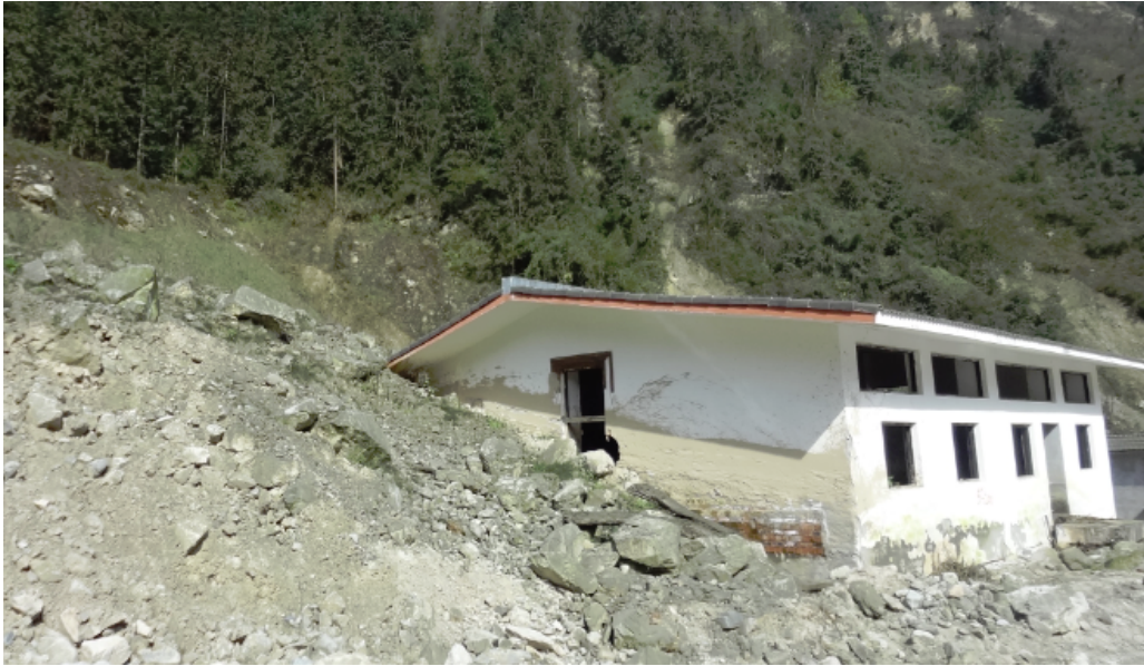
Figure 5.2 Landslide damage in Sichuan, China, 2010
