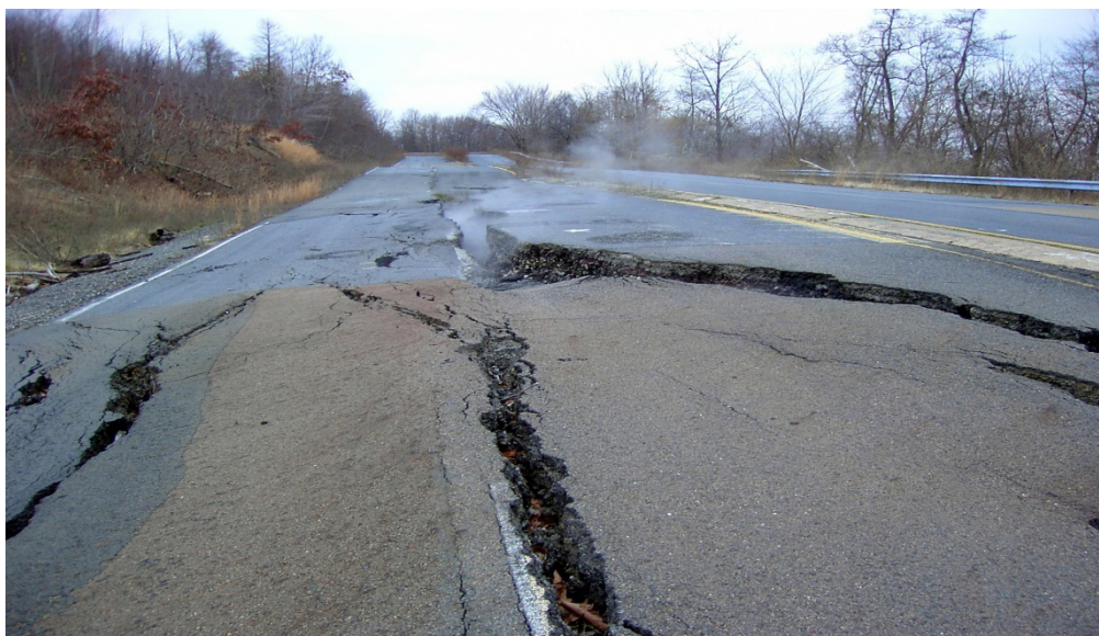
Plate 12.2. Damage to a road surface near Centralia PA due to the anthracite fire.
