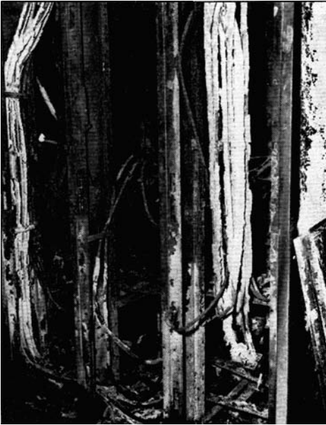
Figure 1 Burndown damage caused by arcing fault. View shows low-voltage cable compartments of secondary unit substation
