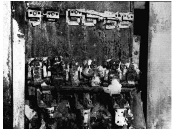
Figure 3 Fused feeder switch consumed by arcing fault in high-rise apartment main switchboard. No intermediate segregating barriers had been used in construction
