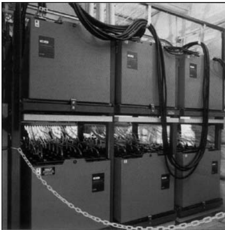
Figure 6 Large lead-acid battery bank
