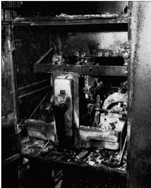
Figure 4 Remains of main secondary circuit breaker burned down during arcing fault in low-voltage switchgear section of unit substation
