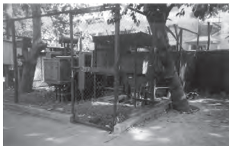
Fig. B59: Outdoor substation without enclosure
