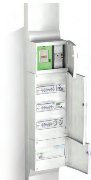
Fig. Q4 : Control and distribution board
